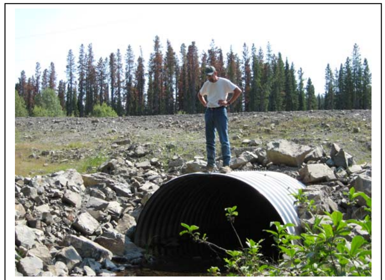
Photo #1: Pro active approach. Apollo has been completing Fish Habitat Assessments on suitable candidate creeks and replacing smaller corrugated metal culverts with open bottom plate arch culverts to allow fish passage to habitat upstream. This arch is located on Leo Mainline. Note the dead pine in the background.
