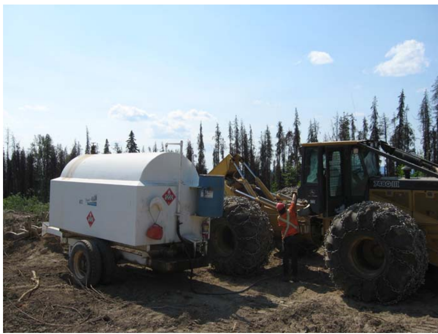
Photo #2: A Contractor is visited as part of the audit process. In addition to interviewing Workers to determine their level of environmental awareness, work habits are observed. An operator fuels his machine from a mobile double walled enviro fuel tank. Note the unit has the appropriate signage, posted fueling procedures, an inspected fire extinguisher and adequate spill response kit (blue barrel). There is also containment for the fuel nozzle once the operator is finished.
